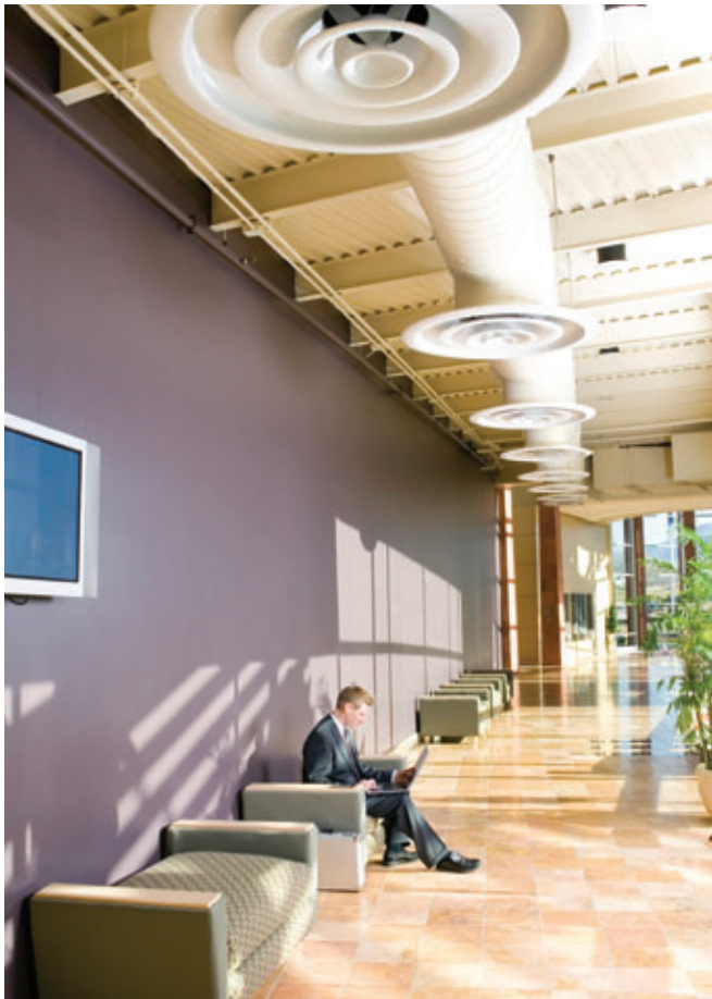
Some fabricators of HVAC equipment use antimicrobial coatings in air-handling ductwork as a defense against indoor air contamination. Photo courtesy of Sureshield Coatings Company.
