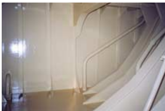
A light-coloured coating, such as on this fresh water tank, is an aid to effective inspection.
