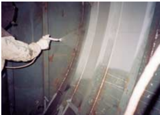
Ballast tank protection is critical to a ship's service life. This coating is being applied to the fore peak tank.
