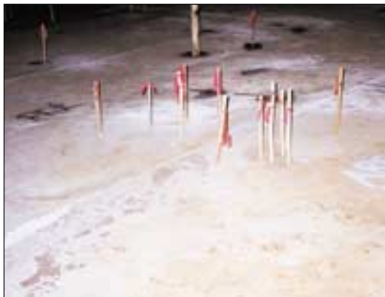
Fig. 7 - Numerous holes found by MFL/EC in lined tank bottom. (Note: Wooden stakes inserted into holes as location markers.)
