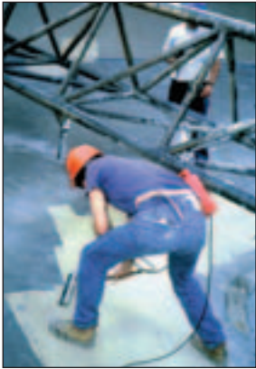
Holiday detectors can find coating defects that may not be visible
