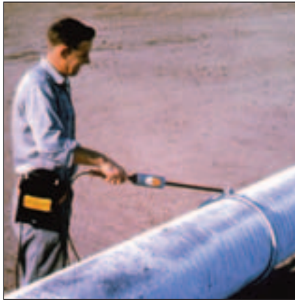
Fig. 3: Performing holiday detection on a pipeline with a full-circle coiled spring electrode
