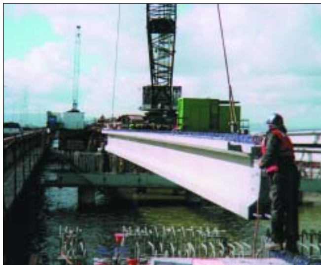
Concrete girder with aliphatic polyurea topcoat being placed on substructure for San Mateo-Hayward Bridge widening project
