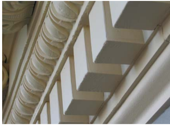
Following removal of paint from the cast-iron elements by means of a composite-sponge blast technique, the surfaces are being repainted using a high-performance epoxy primer and acrylic topcoat system.
