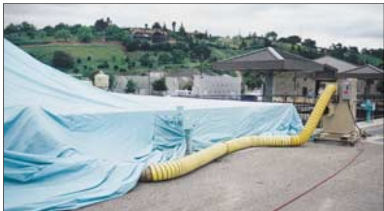
Dehumidification equipment set up at Santa Theresa Water Treatment Plant, Santa Clara, CA Photo courtesy of Munters Corporation, Moisture Control Services
