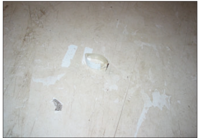
Fig 2: ASTM Tape Test revealed poor coating adhesion
