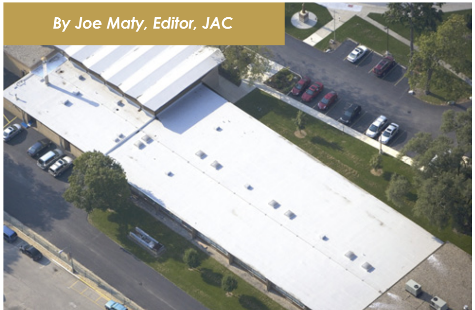
The black EPDM roof of the BVM Maternity school in northern Illinois was restored following Mule-Hide Inc.'s EPDM Restoration System™ program. The program includes preparation of the existing roof with thorough cleaning and repairs, application of a proprietary resurfacing agent to the existing roof to facilitate coating adhesion, and application of a white reflective acrylic elastomeric coating. Photo courtesy of Mule-Hide Inc.
